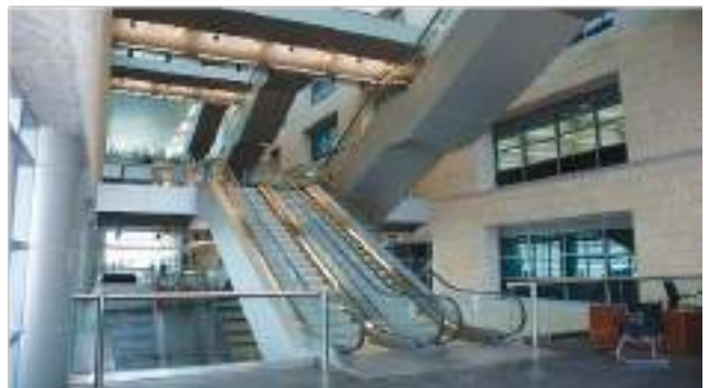
Building Transport Systems
